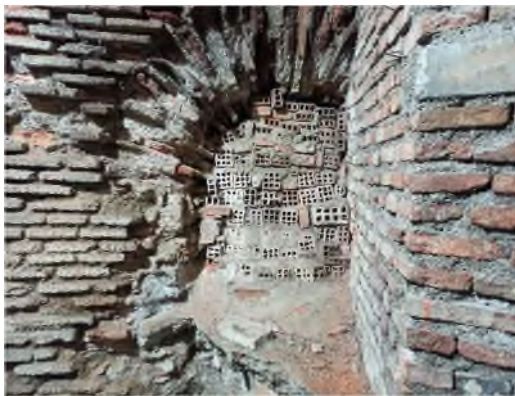
Figure. 10 Degraded masonry observed on wall surfaces.
