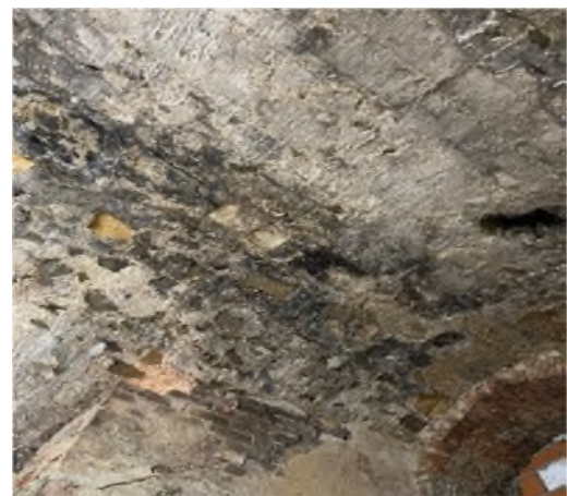
Figure. 6 Black mold growth on the vault surface.
