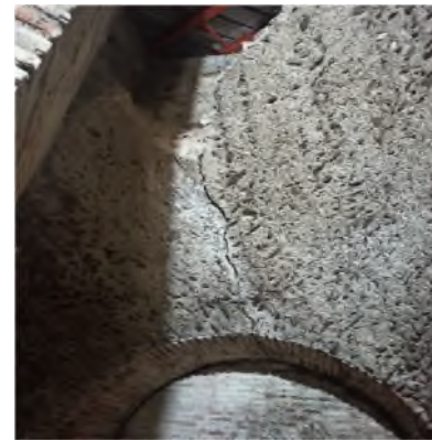
Figure. 5 Crack observed on the interior wall.
