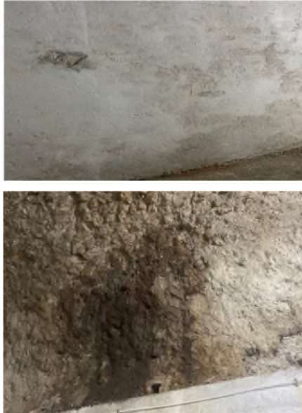
Figure. 7 Moisture stains on vaults and walls.
