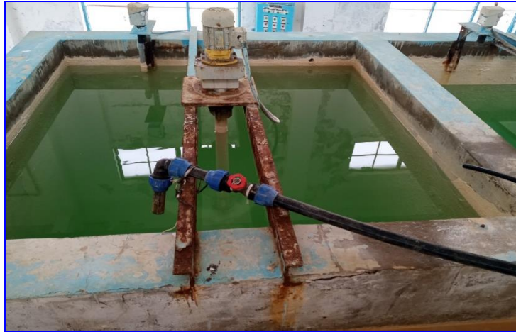
Figure II.10. Salle de chloration.
