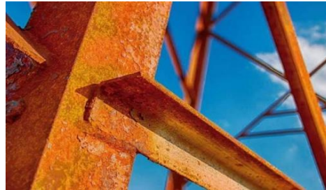
Figure .I.4: la corrosion uniforme
