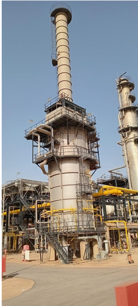
Figure 1.7 the industrial furnace H-231 in train 1
