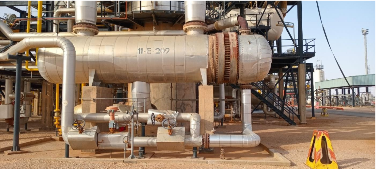
Figure 2.3 train 1 deethanizer's reboiler
