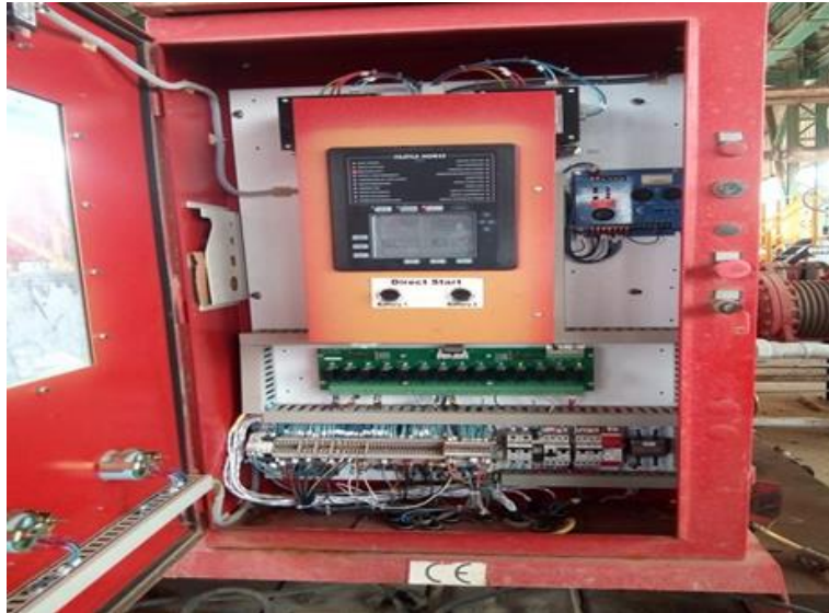
Figure III.11: Station de commande local de la pompe.
