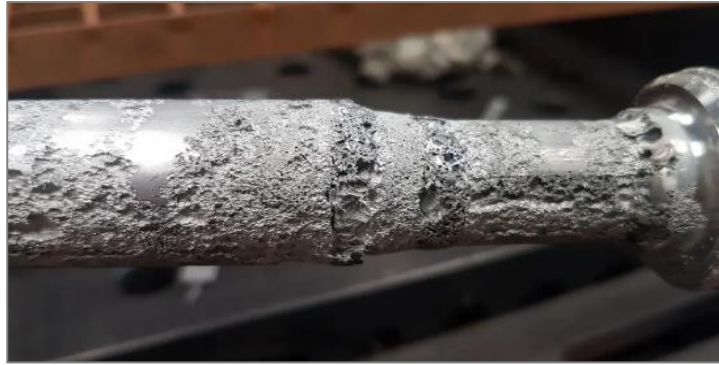
Figure I.8 : Corrosion caverneuse inox
