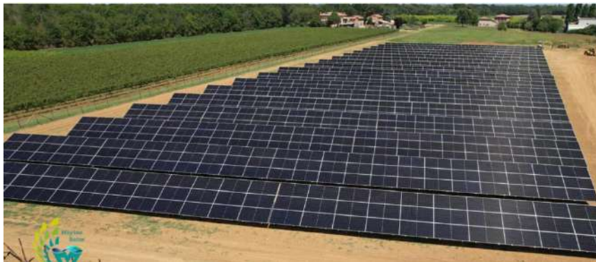
Figure I-5: Photovoltaic solar module.
