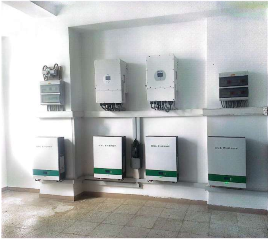
General view photo of two master-slave inverters (upper middle), AC distribution box and DC distribution box (on the left and right of the inverters), and 4 batteries.
