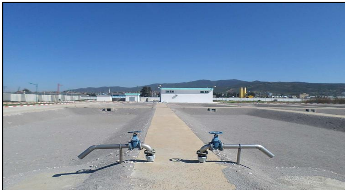
Figure III.21. Lits de séchage.
