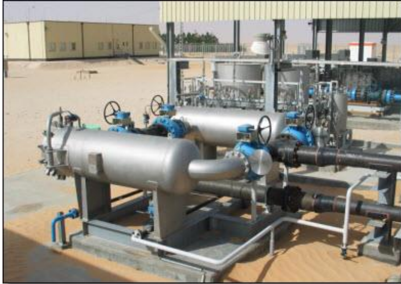
Figure I.19 : Deux Filtres 40-F-201A/B.
