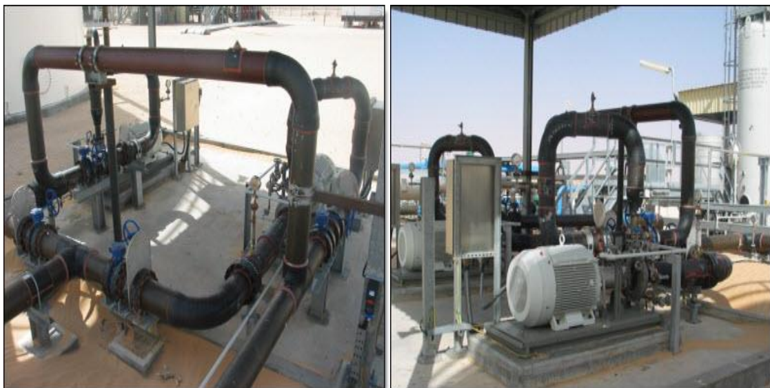
Figure I.18 : Deux pompes BOOSTER 40-P-201A/B.
