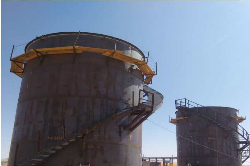
Figure I.5 : Bacs de stockage corrodé.
