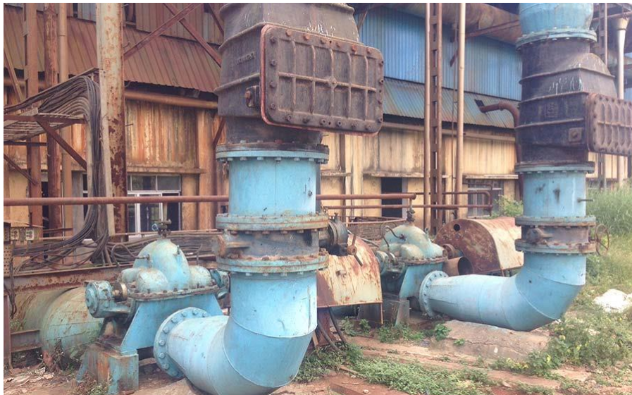
Figure I.6 : corrosion des pompes. [22]
