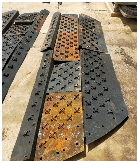
Figure III.8: corroded trays after their collapse.
