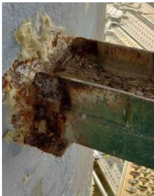
Figure III.6: Tray support corrosion.
