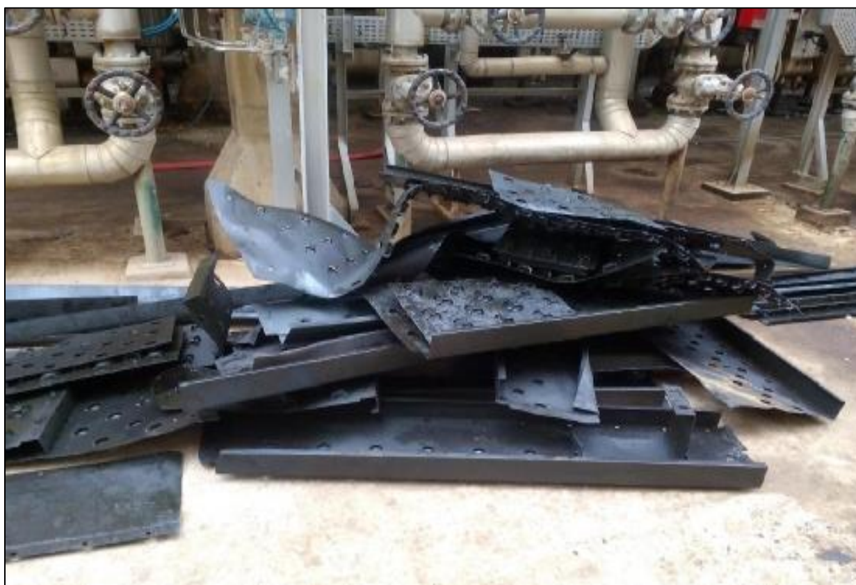
Figure III.9: The state of the C1 trays after a high vapor flow rate that caused their collapse.
