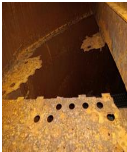
Figure III.7: perforated tray due to corrosion
