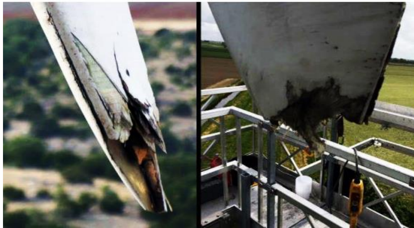
Figure II.10 Wind turbine blade damaged by lightning.
