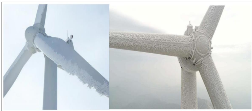
Figure II.11 Ice buildup on wind turbine blades[90].
