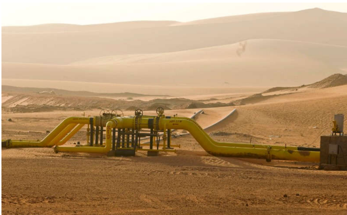
Figure (Photo) IV. 1. Pipeline (gazoduc) BRN – MLE (Champ de Berkine).
