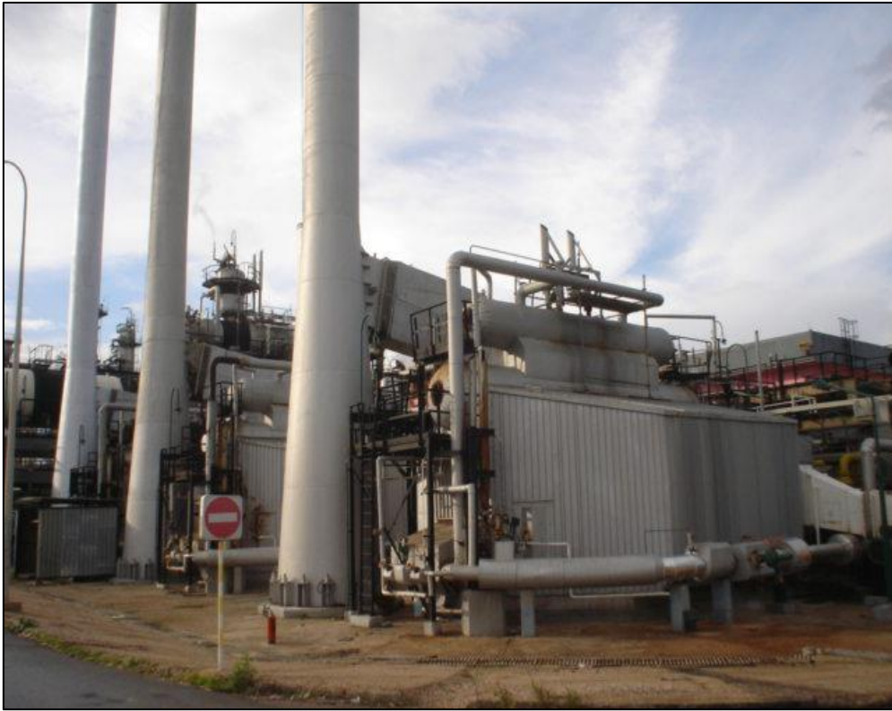
Figure II.16: Chaudière STEIN 51H01/02/03.
