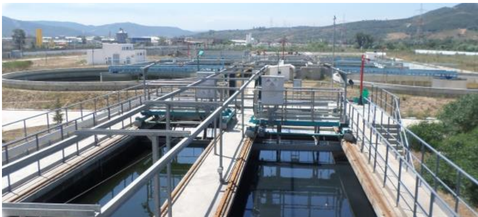
Figure III.13: La station d'épuration de Hamadi Krouma.
