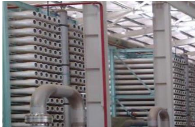
Figure II.5 : Racks d'osmose inverse
