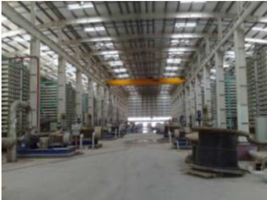
Figure II.4 : station de dessalement
