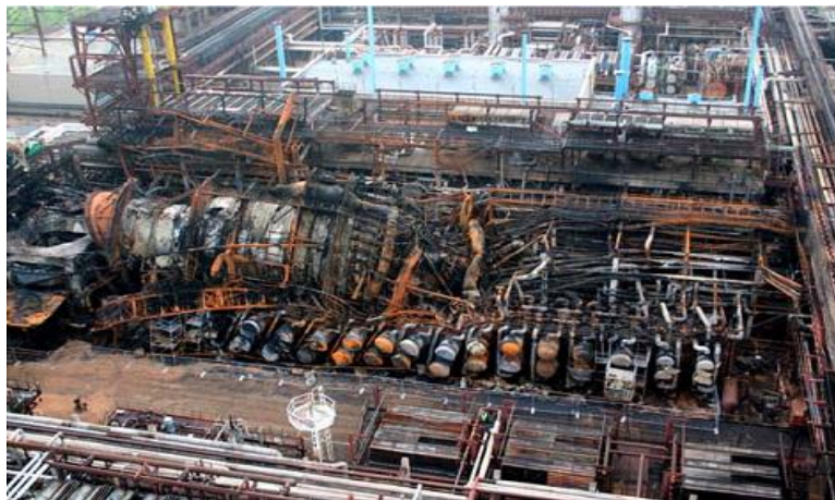
Figure. I.1: Risques due à la corrosion.
