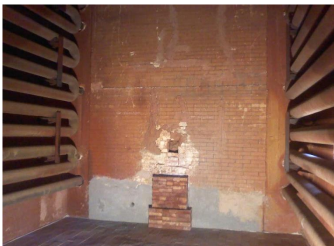
Figure I.3 Serpentins du four Topping.
