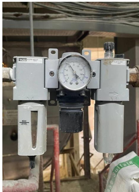
Figure II.25 : Real filter-regulator unit observed in the industrial site.
