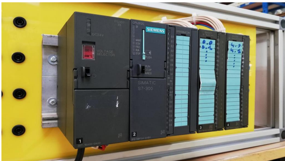
Figure 1-1 : Automate SIEMENS S7-300 [2]
