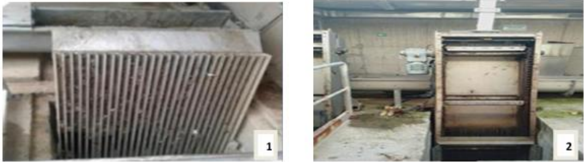
Figure 1.5: Automatic Fine Screen (1) and Manual Fine Screen (2) (Sidi Merouane Wastewater Treatment Plant, 2019)
