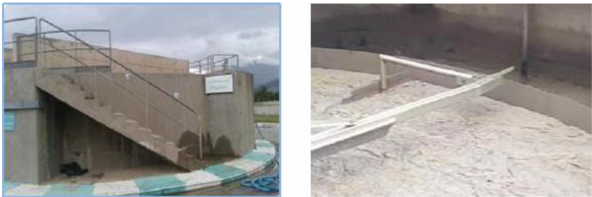
Figure 1.11: Degasser (Sidi Merouane Wastewater Treatment Plant, 2019)
