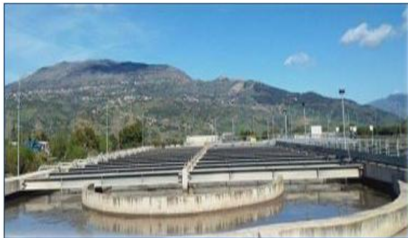
Figure 1.9: Biological Basin (Sidi Merouane Wastewater Treatment Plant, 2019)
