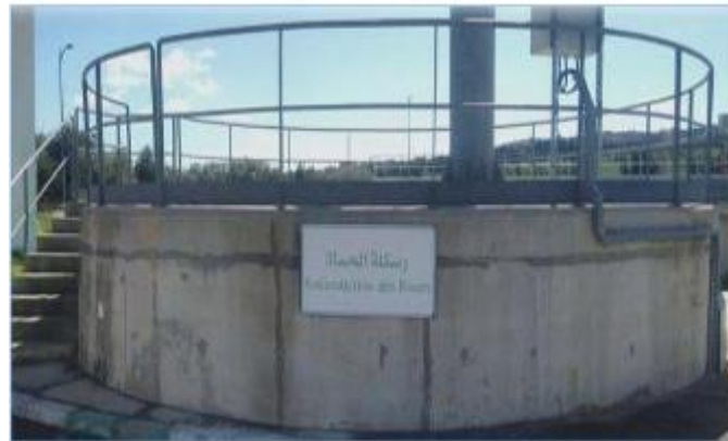
Figure 1.13: Sludge Recirculation (Sidi Merouane Wastewater Treatment Plant, 2019)
