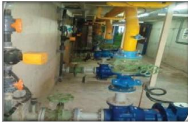
Figure 1.7: Sand Pump (Sidi Merouane Wastewater Treatment Plant, 2019)
