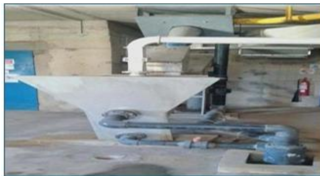
Figure 1.8: Sand Classifier (Sidi Merouane Wastewater Treatment Plant, 2019)
