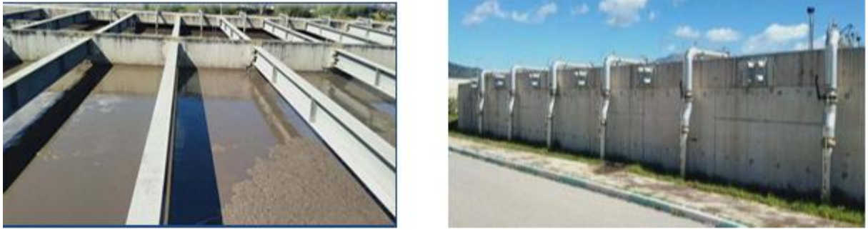
Figure 1.10: Aeration System (Sidi Merouane Wastewater Treatment Plant, 2019)
