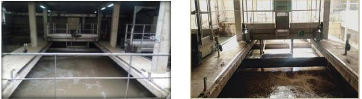
Figure 1.6: Sand Separator and Oil Separator (Sidi Merouane Wastewater Treatment Plant, 2019)
