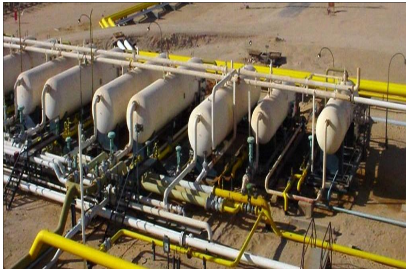
Figure 3.2: Installation for treatment and storage of crude oil
