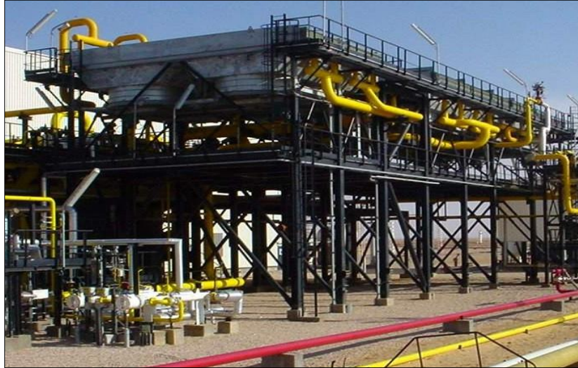
Figure 3.4: Associated Gas Recovery Unit
