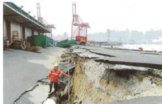
b) Quay wall earthfill Kobe 1995
