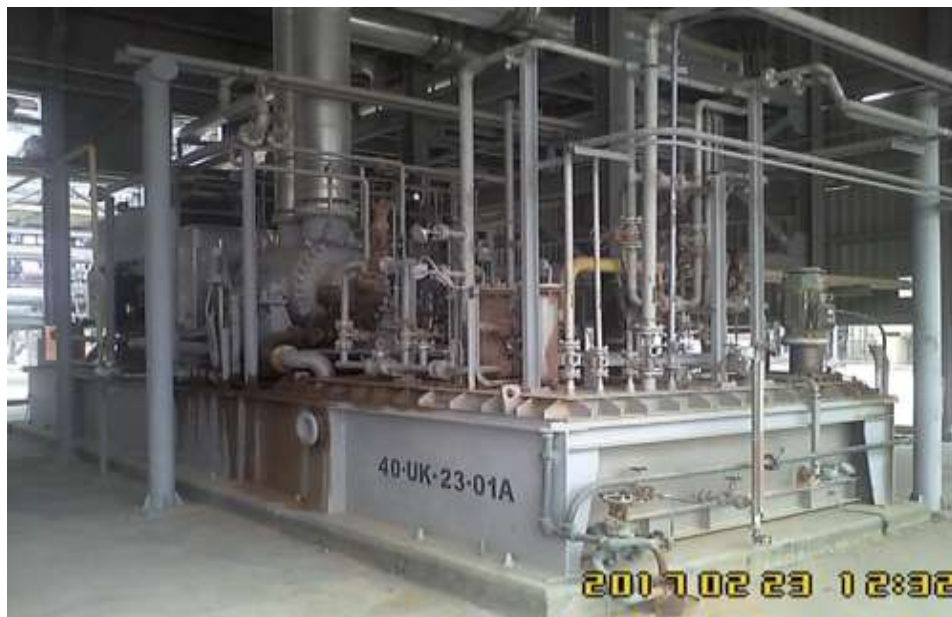
Figure II.12: Stripper OverHead compresseurs.
