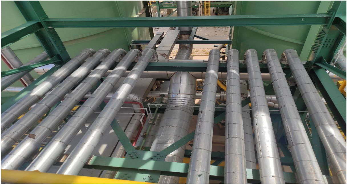
Figure 4.5 les 12 tubes de four 1120-F-1.
