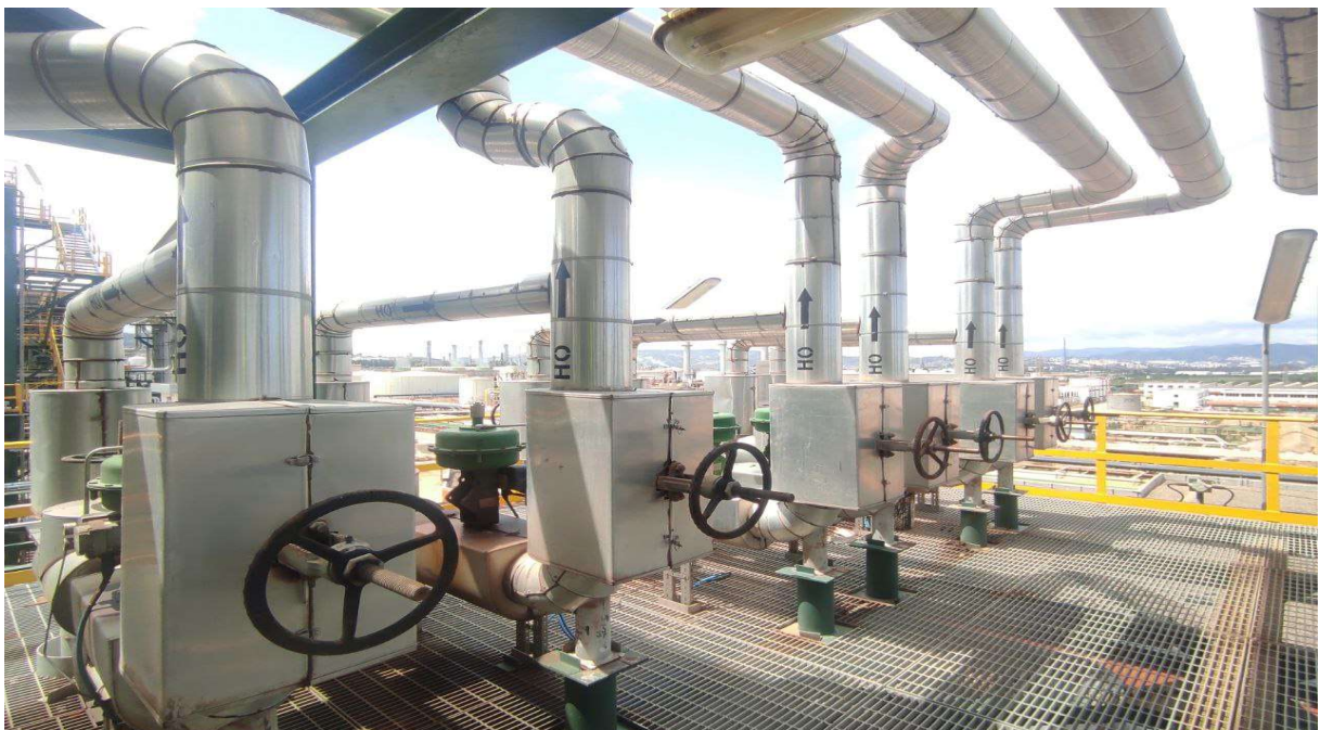
Figure 4.6 6 tubes de chambre A de four 1120-F-1 .
