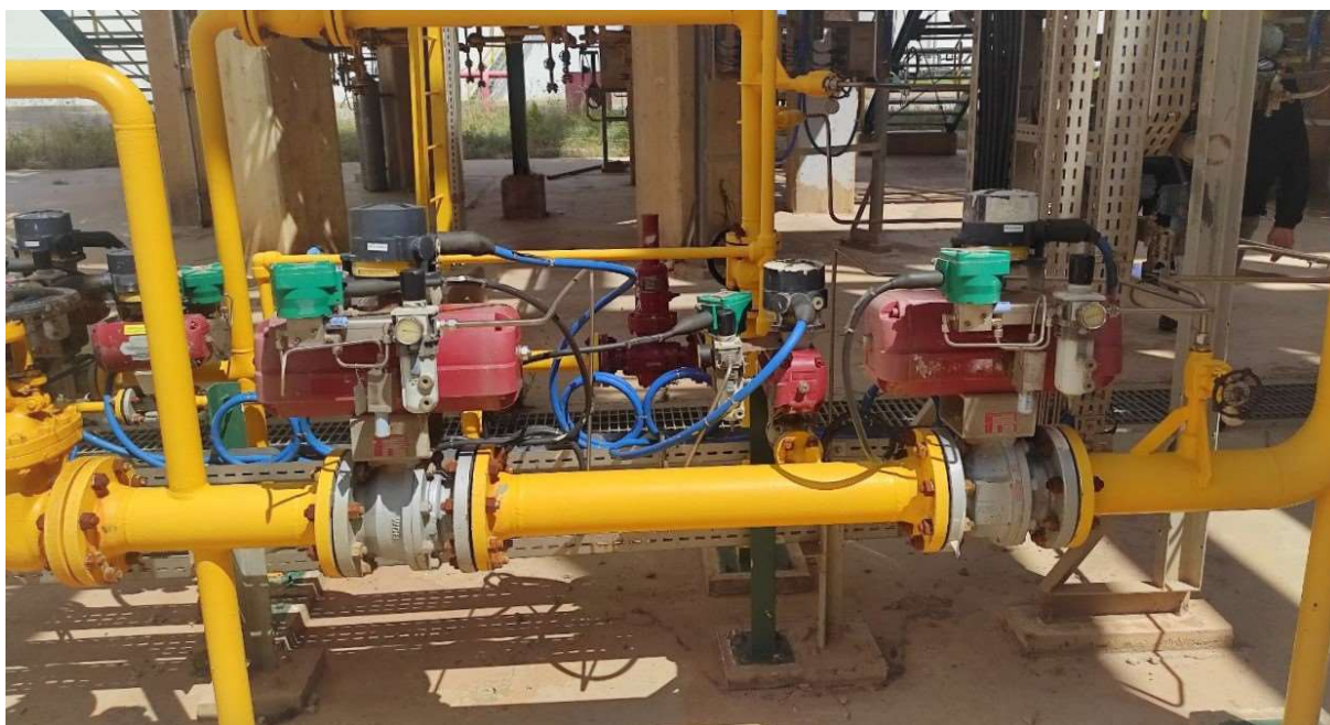
Figure 2.22 vannes de blocage (block valve) .
