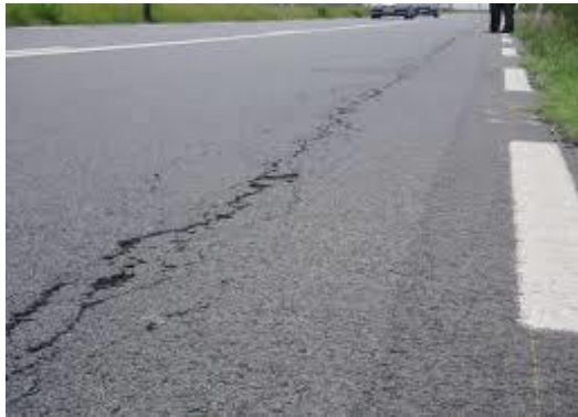
Figure II.8. Fissures du gel [25].
