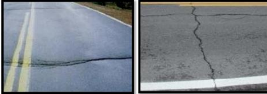
Figure II.4. Types de fissures transversales [31]
