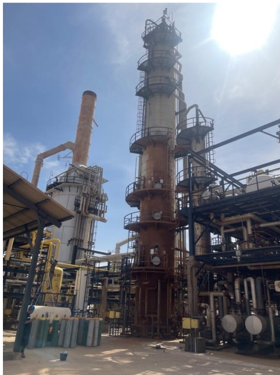
Figure II.15 : Colonne de distillation
