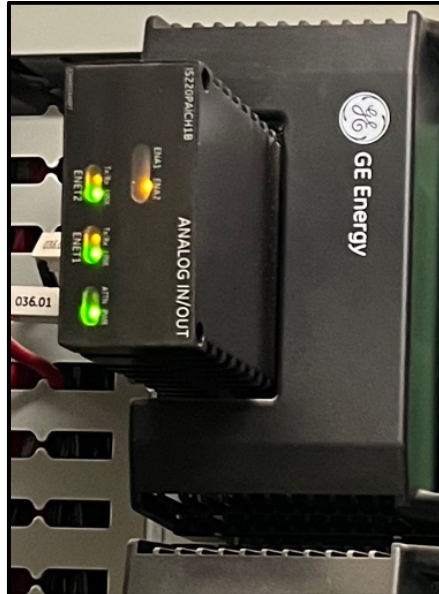
Figure III.2 Les I/O packs.
