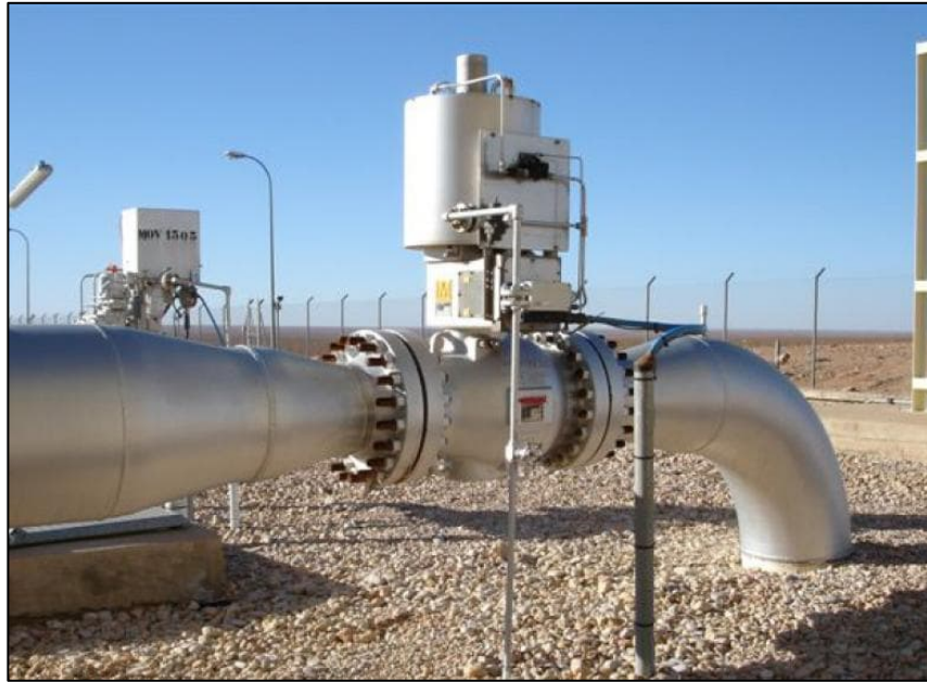
Figure II.25 La vanne anti-surge. [32]
