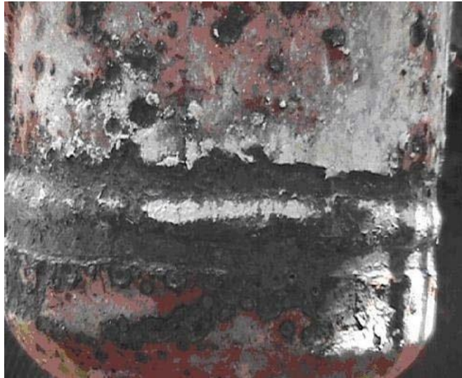
Figure 3.4: Oxidation of the OD of a carbon steel furnace transfer line [3].
