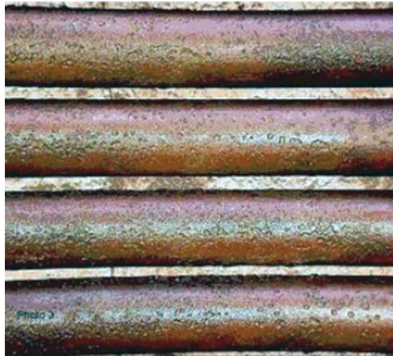
Figure 3.3: General metal loss and pitting of tubes exposed to moisture [3].
