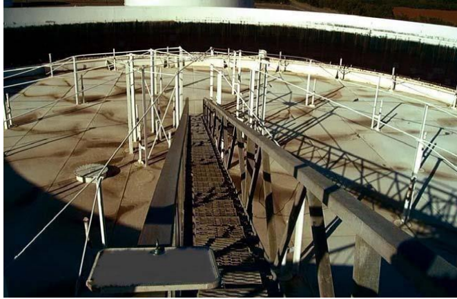
Figure 1.4 Pan-type floating-roof tank [27].
