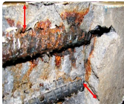
Figure II.17. Effet de la corrosion (Epaufreure).
